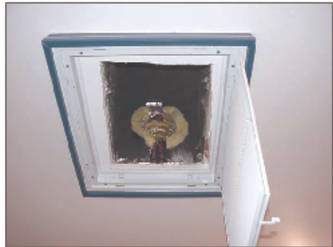
Figure 4.6b — Silent duct boot, grille open
